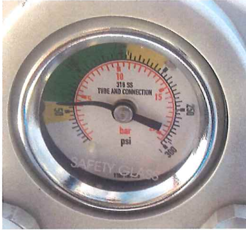
Example of Pressure Gauge damage
