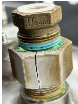
Figure 2 - Cracked CB8426, PRV Adaptor
